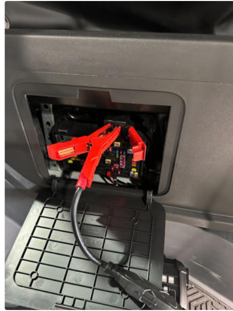
Terminal located at Driver Side Towards Door Opening
